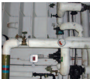
Asbestos insulation on pipes
